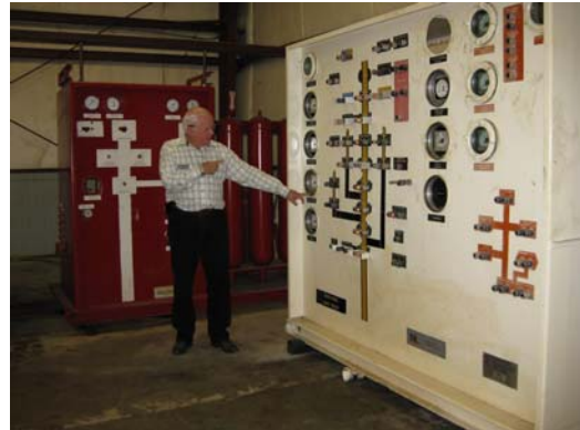
Instructor Conley Perry points out control panel components
